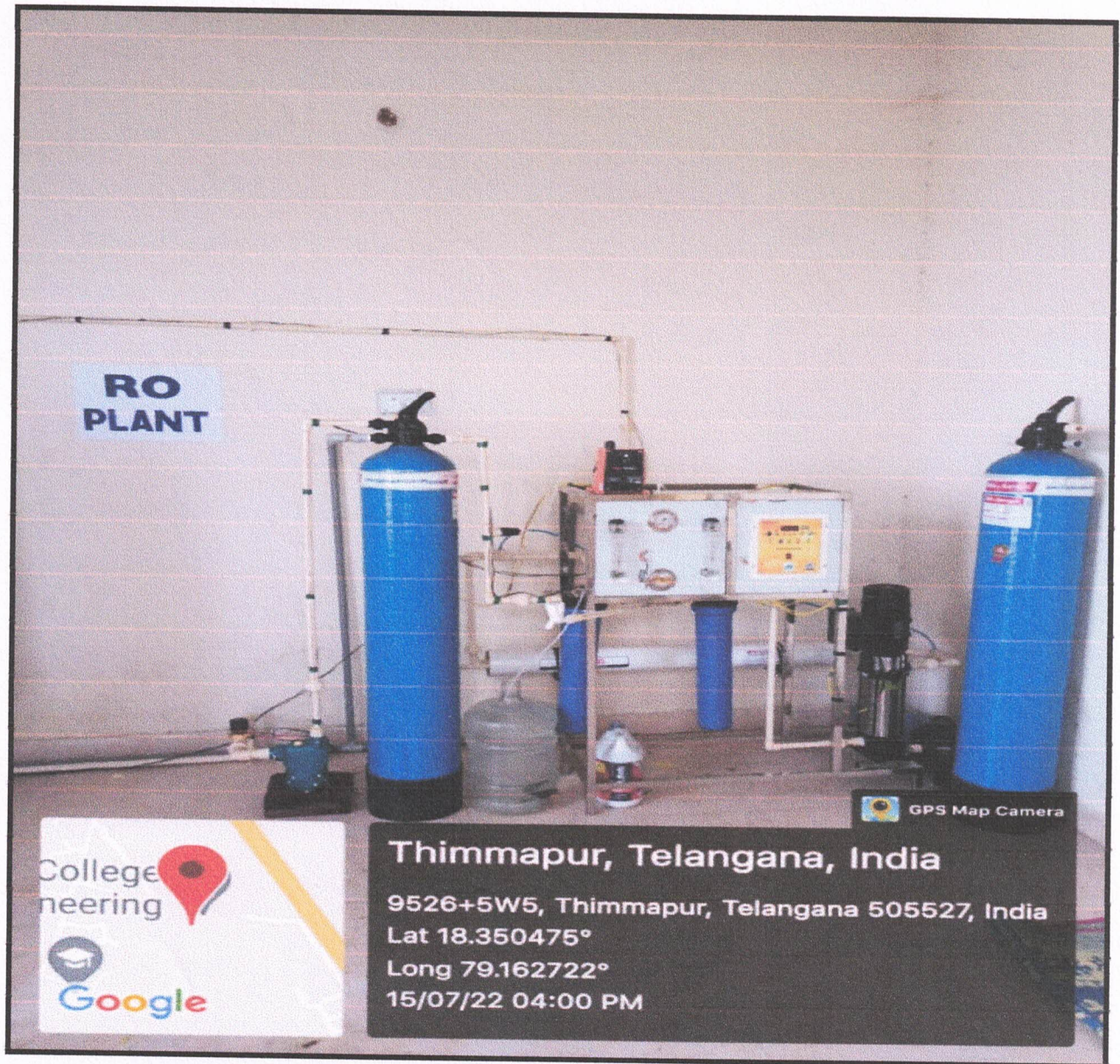
RO plant at VGSE
