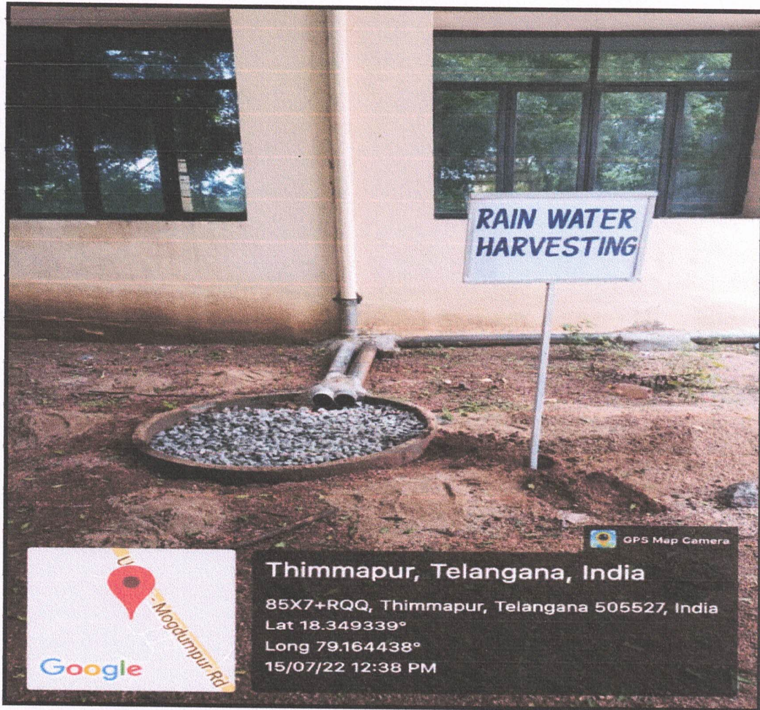
Rain water harvesting pit in open land area
