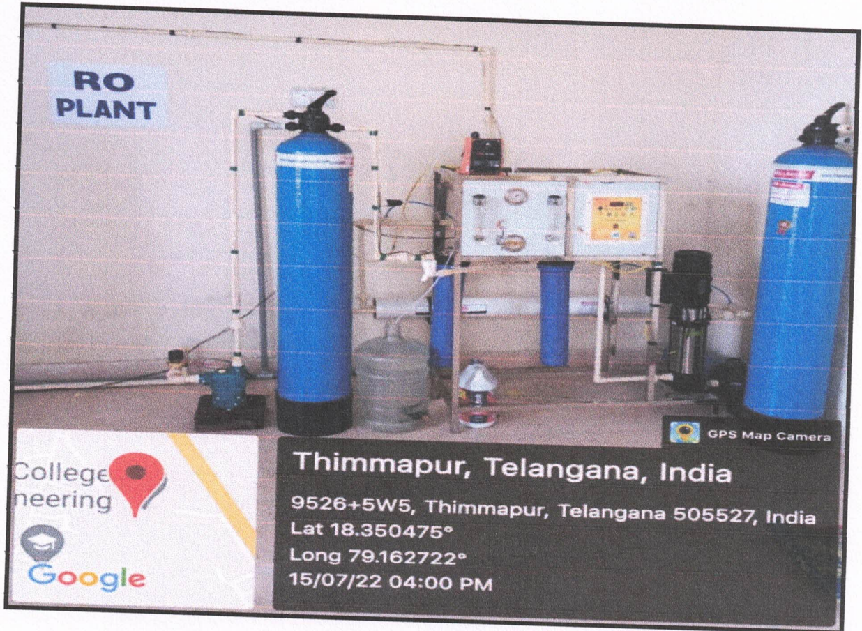
RO Water plant in VGSE
